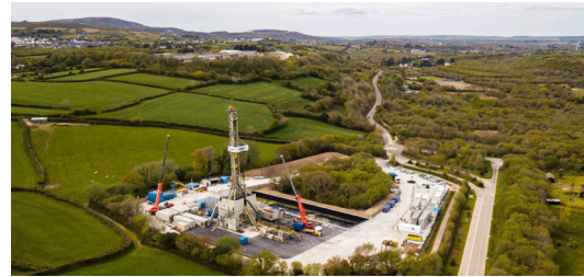
Geothermal Plant at Eden, Cornwall
