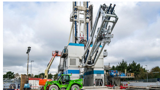
Geothermal Plant at United Downs Industrial Park, Cornwall
